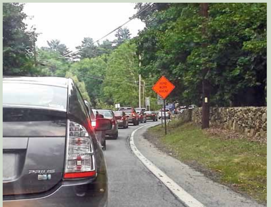
Repair work began June 24 on the stone wall along St. Philip's Church in Garrison. Single lane traffic may cause delays on route 9D.
