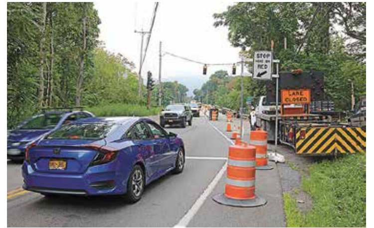
In 2019, the state spent $2.2 million on repairs to the Indian Brook Bridge on Route 9D, which was a single lane for much of the summer.
