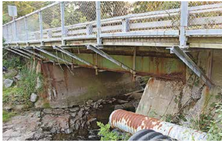
The 86-year-old bridge carrying Sprout Brook Road in Philipstown over Canopus Creek is scheduled to be replaced at a cost of $1.6 million.
