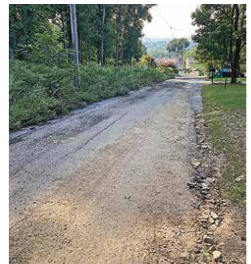
Federal infrastructure money could help Beacon rebuild Pocket Road.
