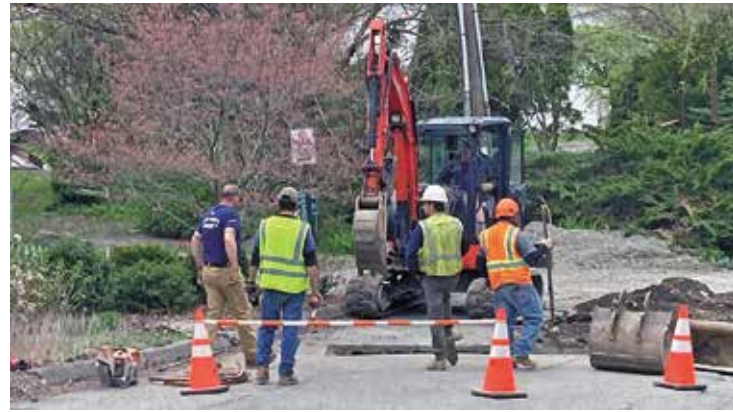
Workers search on Dock Street for the source of a water leak at Garrison’s Landing.
